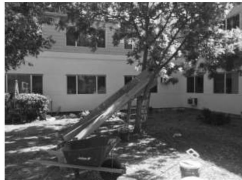
Apartment complex rehab on F - no tree protection fence at construction site required by policy.
