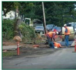
As pavement conditions deteriorate, maintenance and repair costs become increasingly more time intensive and costly.
