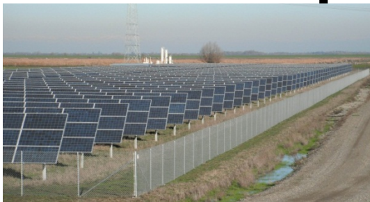
Solar Panels at the Wastewater Treatment Plant
