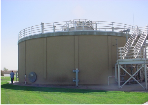
Digester at the Waste Water Treatment Plant
