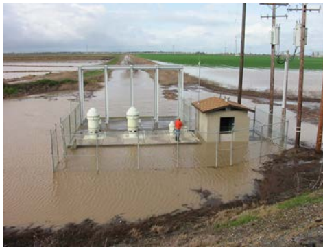
Storm Drainage Station #5
