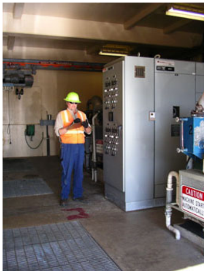
H Street Storm Drainage Station
