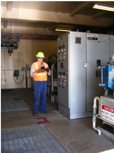
H Street Storm Drainage Station
