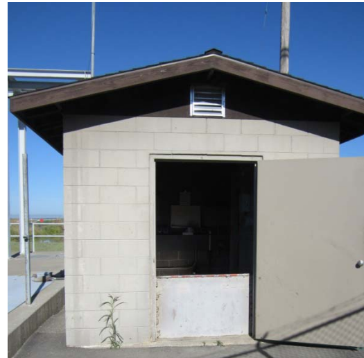
Plate across building door
