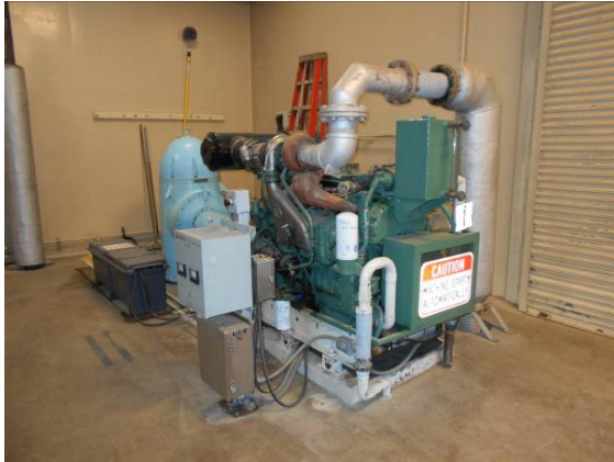
Typical stormwater pump
